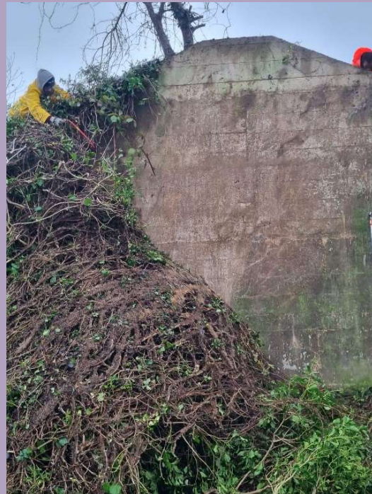
Removing ivy from a wall at the Gorse Industrial Estate, a Historic England site.
